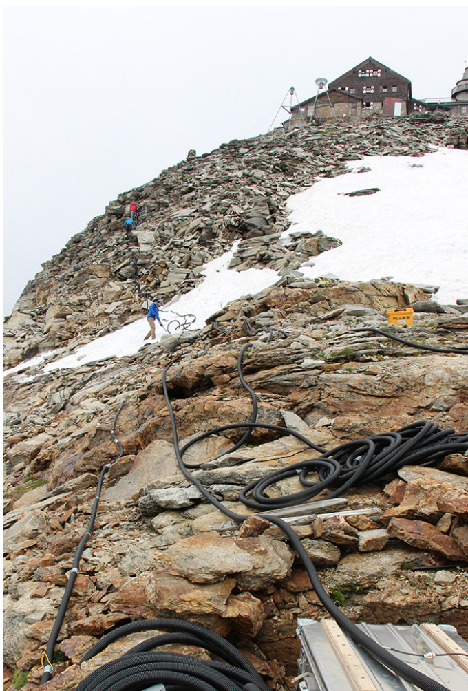
Figure 4. Installation of an ERT array in the summit area of Hoher Sonnblick (3106 m asl.) on 14 July 2015. The Sonnblick Observatory and the summit hut Zittelhaus are visible in the background. Photograph provided by Stefan Reisenhofer.
