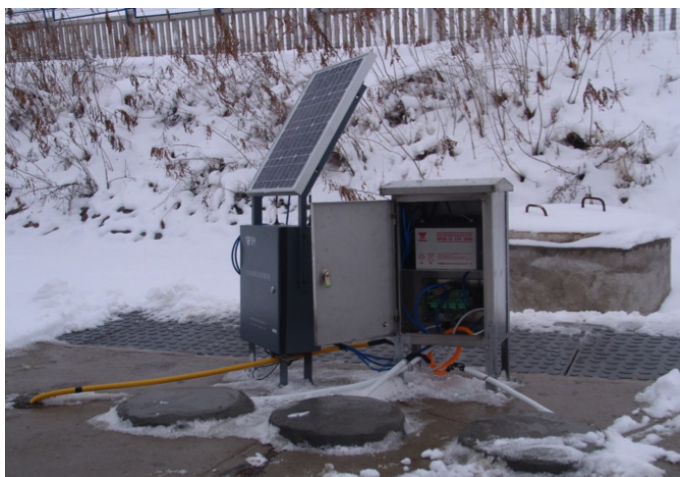
Figure 3. A ground temperature and deformation monitoring site along the HDR. The yellow tube with temperature probes inside is for ground temperature monitoring; the concrete plates with white tubes are for deformation monitoring. The data are collected by datalogger and accessed remotely in Lanzhou.
