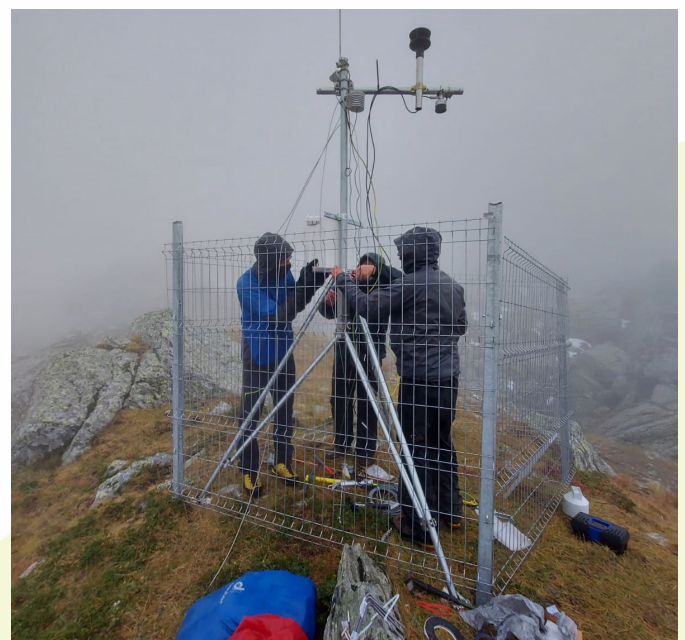
Fig. 54. Installation of the automatic Campbell Scientific meteorological station on Căldarea Pietroasă cirque. Photo: Alexandru Onaca.
