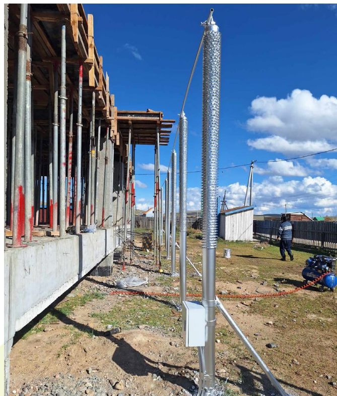
Fig. 37. Foundation with open crawl space and inclined thermosyphons in Arbulag soum, Hovsgol province, Northern Mongolia.
