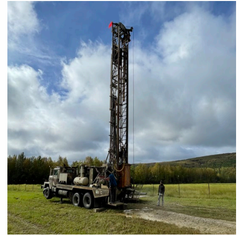
Drill rig being used to drill deep boreholes at farm sites in Fairbanks, AK.
