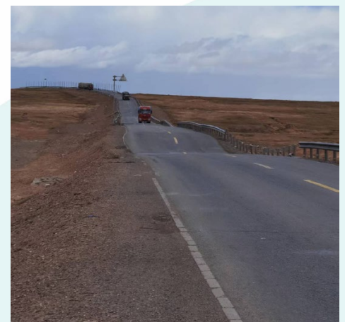
Thaw settlement along the QTH.
