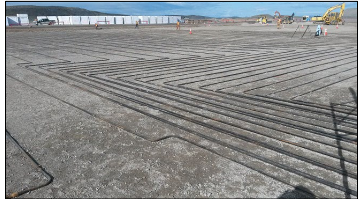
Figure 3. Evaporator installation at the ATB. Rigid insulation is stockpiled in the background.
