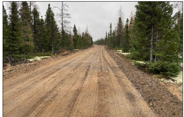
Figure 9. Existing FSFN community road located on a beach ridge north of the airport.
