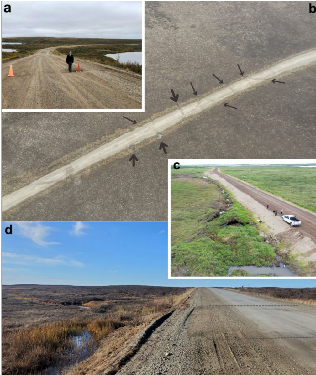
Figure 1. ITH right of way and road surface disturbances. (a) km 100: A linear depression and sinkhole caused by ice wedge thaw and surface subsidence. (b) km 46: An aerial view of ice wedge subsidence beneath the highway embankment, with the thin arrows indicating degraded troughs and thick arrows indicating degraded troughs with ponds at the embankment edge. (c) km 106: Ponding, embankment sloughing, degrading ice wedges, and a heaved mat of organic materials from a large icing and frost blister that developed in the winter 2020/21. (d) km 94: Ice wedges beneath the road expressed as subtle linear depressions, indicated by grey dashed lines, and associated degradation and ponding of ice wedges adjacent to the road. Photos by GNWT – Jurjen van der Sluijs, August 2022 (a), Aurora College – Celtie Ferguson, September 2023 (b), and June 2021 (c), and Aurora College – Jen Humphries, September 2023 (d).
