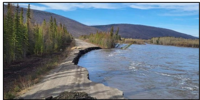
Figure 6. Road washout at km 237 on the Dempster Highway, May 2023. Photo by O. Didier.
