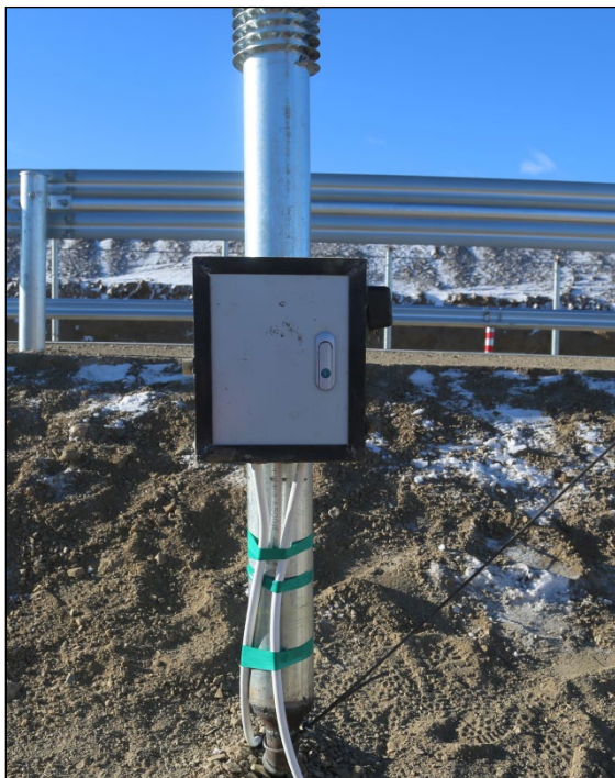
Figure 4. Monitoring box: temperature sensors are installed in white PVC tubes at the end of the evaporator tube and between the thermosyphons.
