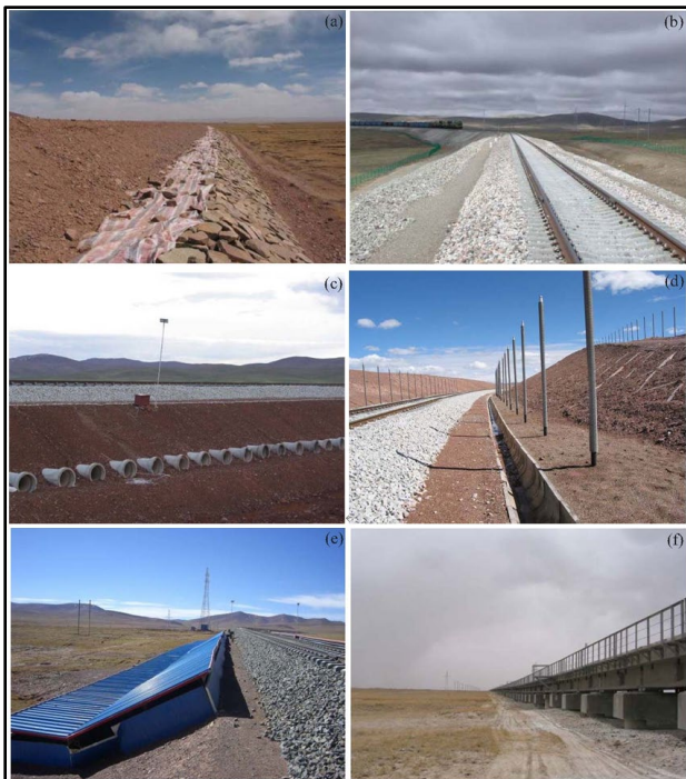
Figure 1. The cooling embankment structures used in Qinghai-Tibet Railway.
