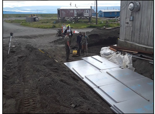
Figure 4. Quinhagak community members and ANTHC extending the rigid subgrade insulation around the perimeter of the structure.
