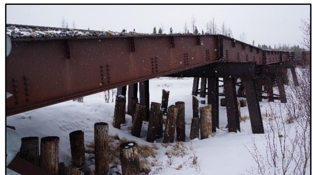
Figure 2. Horn Creek Crossing on the Hudson Bay Railway with 0.5 metres of frost jacking present on the northern pier of the bridge with Span 1 in the foreground pre-repairs made in July 2022.
