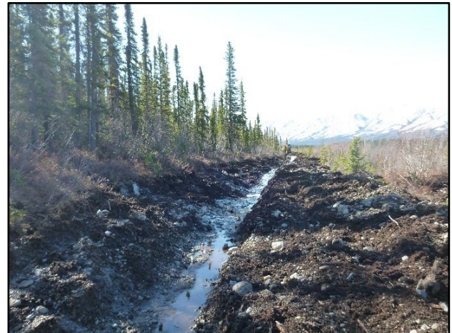
Figure 2. Interceptor ditch located few meters upstream of the Alaska Highway south of Dry Creek, Yukon, Canada. This is one of the drainage methods currently used to keep permafrost degradation that could occur following a ditch construction away from the embankment (Photo: Loriane Périer, 22-05-2013).
