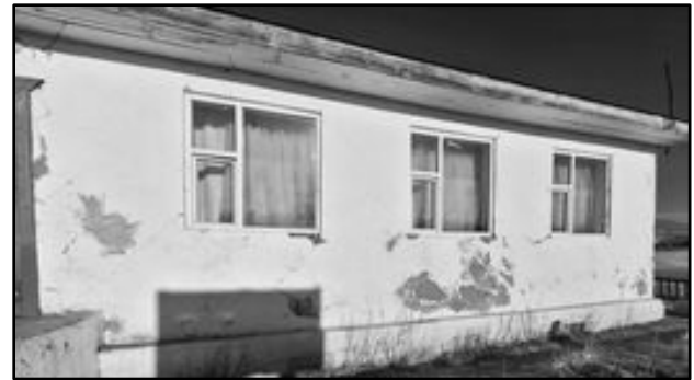
Figure 1. Wooden building in Arbulag soum. The holes in the foundation are for ventilation. Cracks appeared on both the internal and external side walls.
