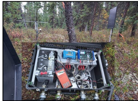
Figure 1. A-ERT monitoring system installation at the MP 788 site near Teslin, Yukon. The A-ERT box contains the 4POINTLIGHT_10W resistivity meter connected to a solar-panel-driven battery, multi-electrode connectors, and a satellite datalink. Electrodes (buried in the ground), the solar panel, and the satellite antenna are all connected via buried cables to the A-ERT box using mil-rated connectors. For additional details on the previous version of this setup, refer to Farzamian et al. (2020).
