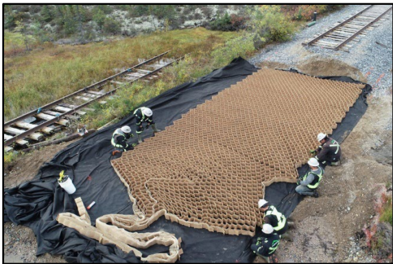
Figure 1. Set up of geocell layer over the HBR railway embankment foundation (Paradox 2021)
