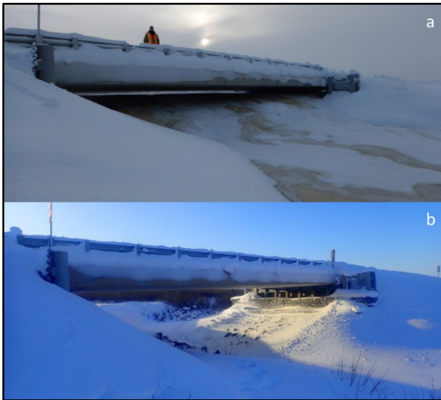
Figure 1. ITH km 8 bridge (a) with aufeis on 25 Feb 2017, and (b) without aufeis on 26 Mar 2022.
