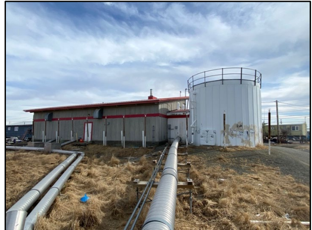
Figure 1. The original thermosyphon system installed at the water treatment plant in Quinhagak, AK, as seen in 2022.
