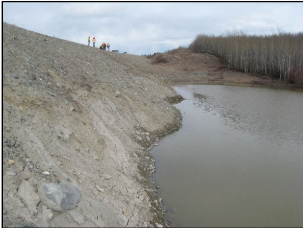
Figure 1. Unstable embankment slope due to water ponding at the embankment toe following the blockage of the culvert by ice at km 1462 of the Alaska Highway, Yukon, Canada (Photo: Benoit Loranger, 05-05-2011).
