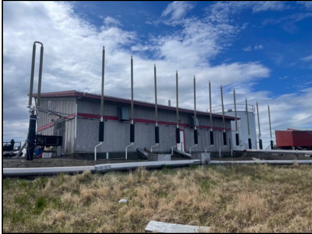
Figure 2. Upgraded thermosyphon system at the water treatment plant in Quinhagak, AK.
